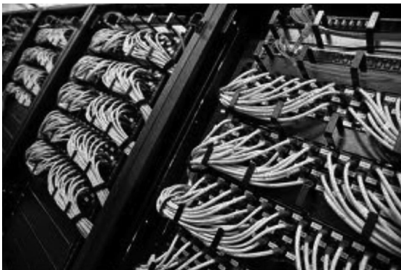
FIGURE 10.2 Networking infrastructure in data centers.
